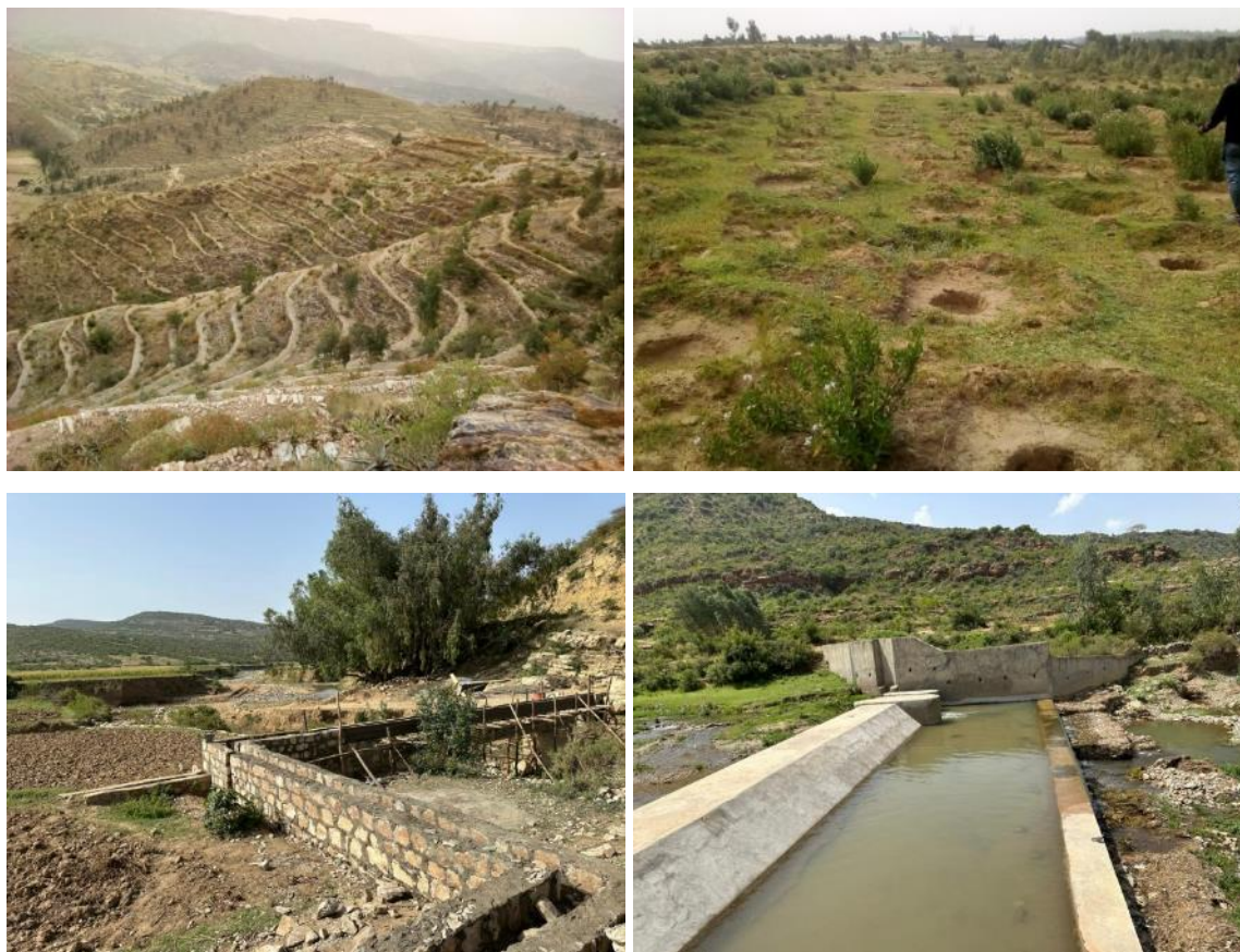
Figure 3: SELAM 1 outputs. Clockwise from upper left: Terracing in Beleso Watershed, water conservation structures in Dimolo watershed, head structure rehabilitation and associated irrigation canal rehabilitation in Tsirea Womberta. June 2023
