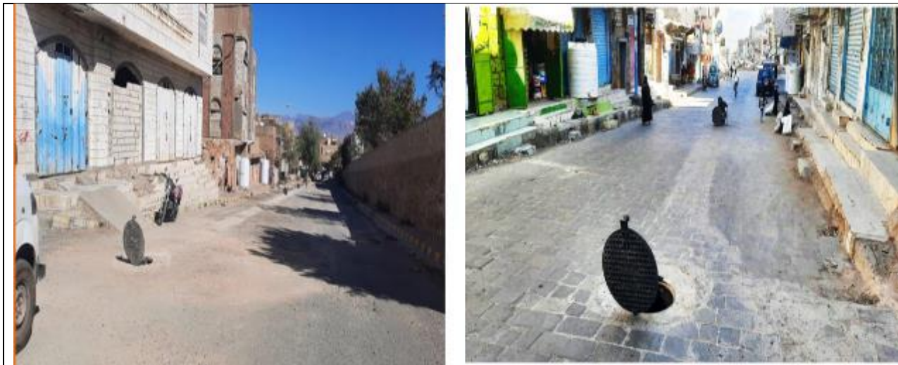
Rehabilitation and replacement of the sewage networks and manholes, Next to the LWSC building , Hawd Al Eshraf sub-district, Al Qahirah district, Taizz governorate
