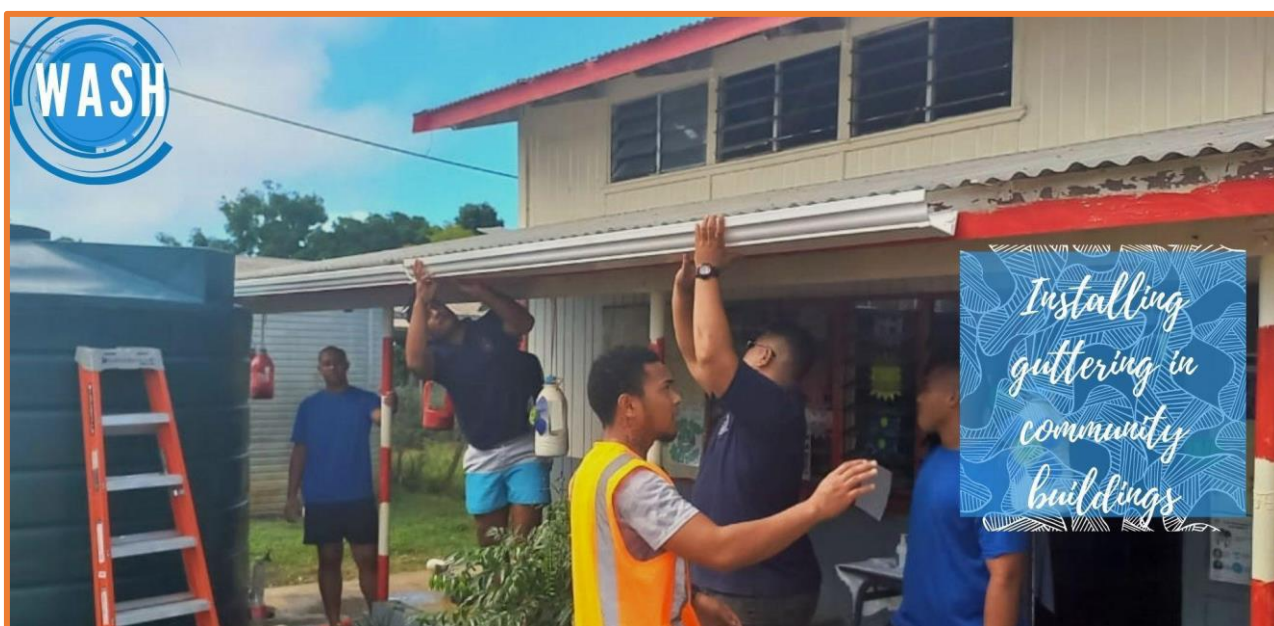
Image 2: Rainwater harvesting system set up at Government Primary School in Fatai. Photo Source: MORDI Facebook Page
