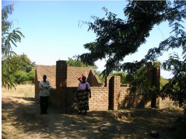
A CBCC structure at Mpokonyola FBO in Chikwawa being supported by a local village donor – 03/06/2008
